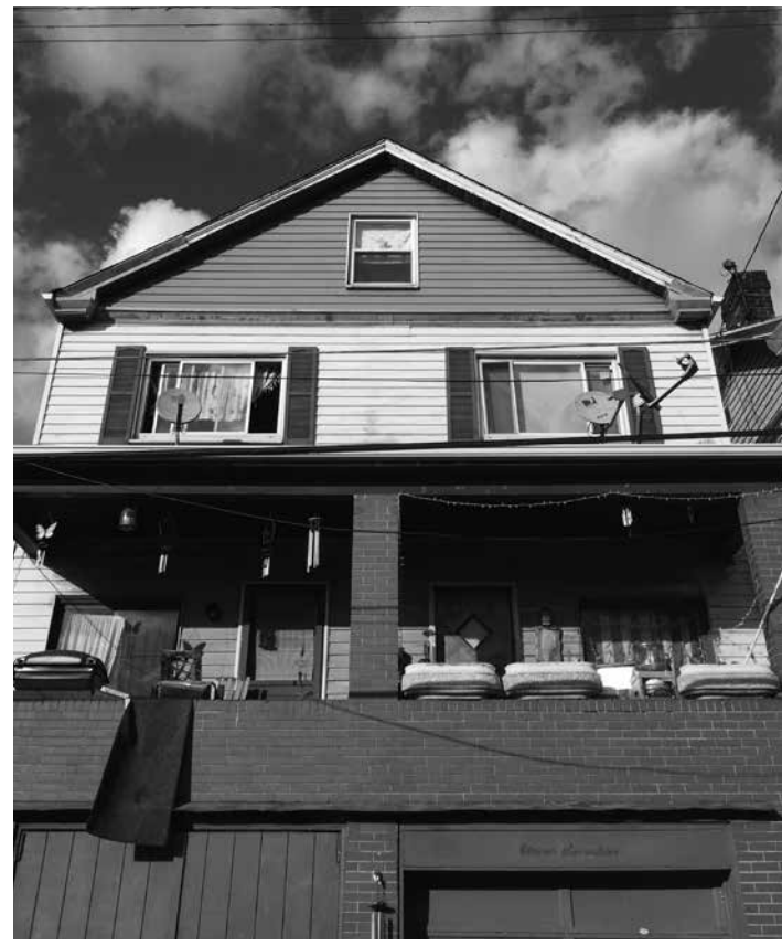
This is Charles and Sharon's property. They live on the right side of the double. The left side has water damage due to a break in the city's water pipe. They are in dispute with the city's water company in regards to who is responsible for the fixing the pipe, and associated the water bills. An example of how these contracts hurt their family: all of the responsibilities of homeownership without the guarantee of owning the home.
