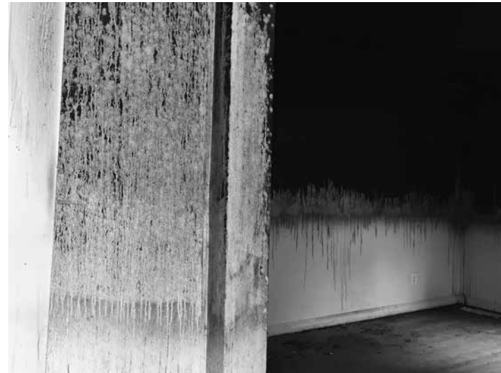
This Detroit property shows the signs of a terrible fire. It appears to have happened while the property lay vacant.
